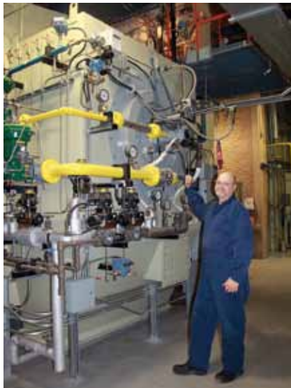
Scope 1 emissions are mainly related to the production and distribution of steam in the Heating Plant, where natural gas is used to generate steam. This is Charles Krikau, shift engineer 2 nd class, with one of six boilers used to produce steam in the Heating Plant.
